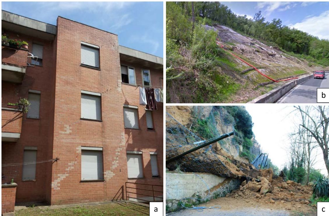
Figure 8 (a) Landslide impacts on building facade; (b) Translational slide affecting the provincial road SP15; (c) Fall within Balze crags area.
