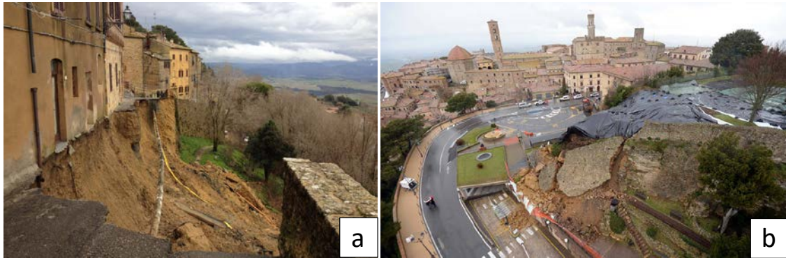
Figure 2 Failures occurred on the Volterra city center: (a) Wall collapse on 31 st January 2014; (b) Wall collapse on 3 rd March 2014.
