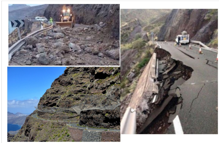
Figure 22. The GC- 200 road between the localities of Agaete and Aldea. It is considered one of the most hazardous roads in Europe. Numerous rockfalls cut the road off every year.
